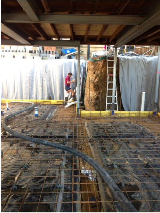
The slab ready for pouring. Note that the Capiphon has been covered with more coarse sand and plastic sheeting before the reinforcing has been laid.
