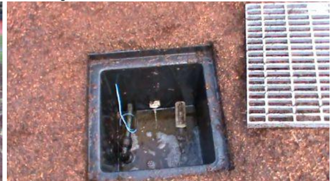
Figure 15. Water flowing from the Capiphon pipe system (left) and the belt system (right) two hours after the rain.
